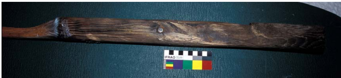
SW face of the flagpole showing the extent of wood loss at the roof line junction and the physical protection afforded by the former metal fitting at the upper part of the pole
