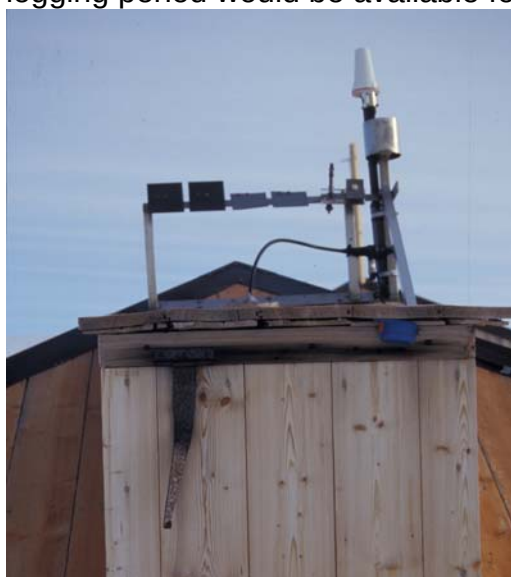
Tinyview logger under ventilator eave
