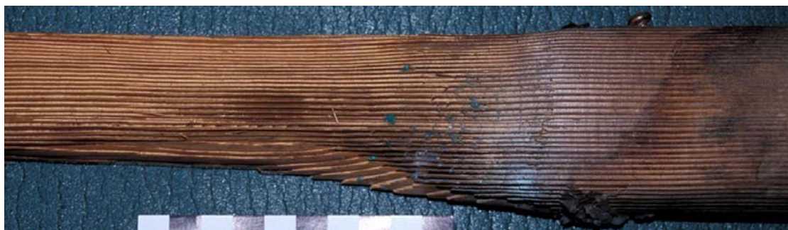
Flagpole showing areas of recent loss and abrasion from SE face
